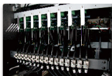
Negative Pressure System
